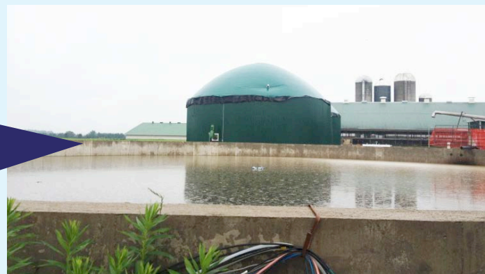
Anaerobic digester with methane trapped under the dome cover.
